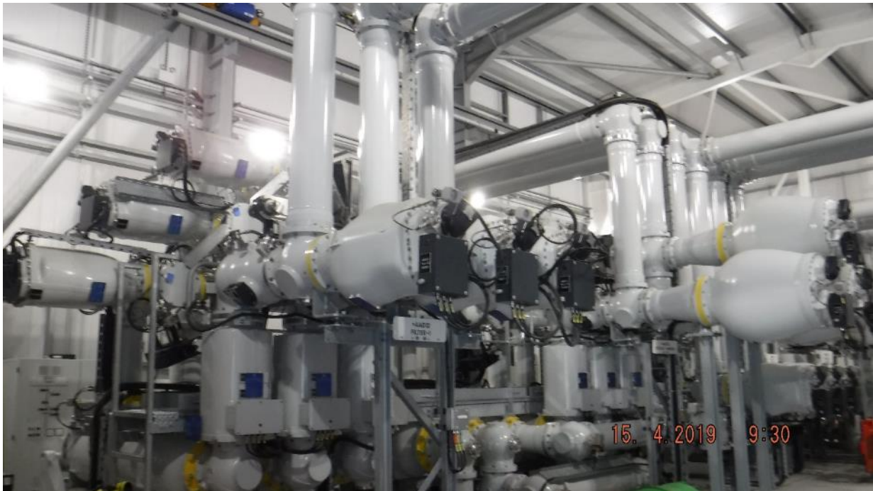
Plate 6.24 Electrical Equipment Contained within the Main GIS Building (example taken from East Anglia ONE substation)
