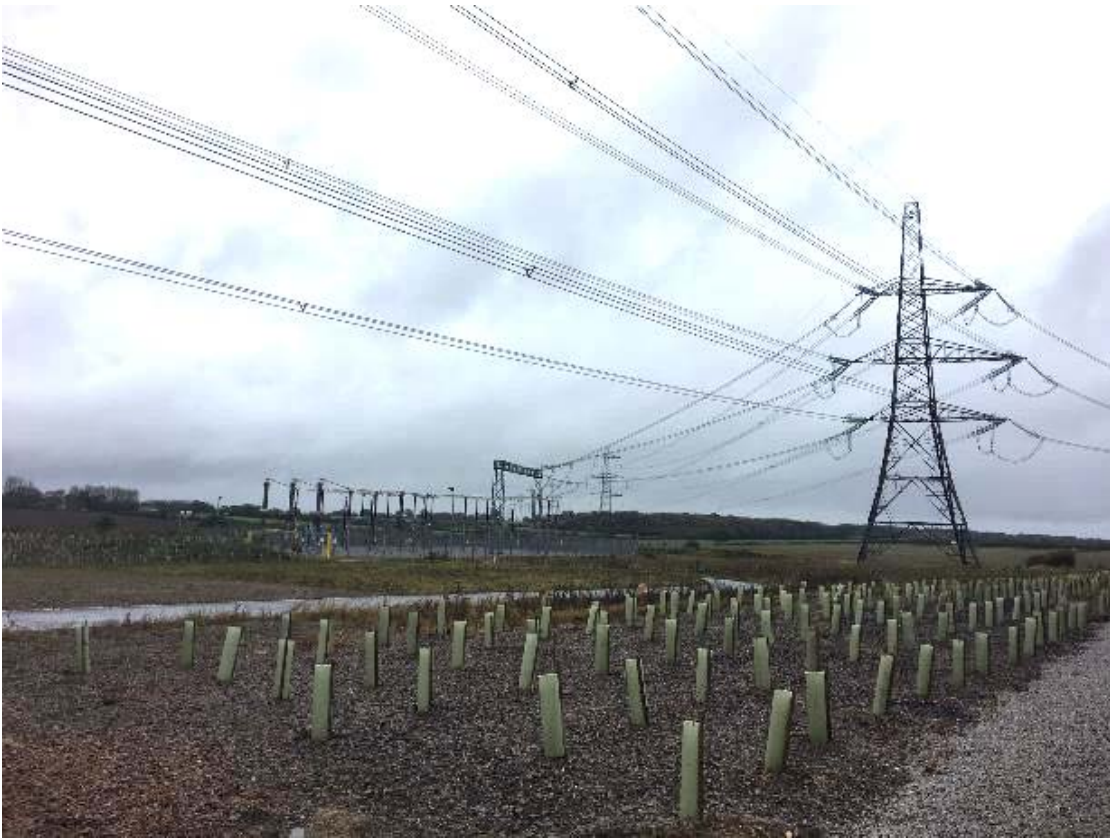
Plate 6.31 Example of cable sealing end compound
