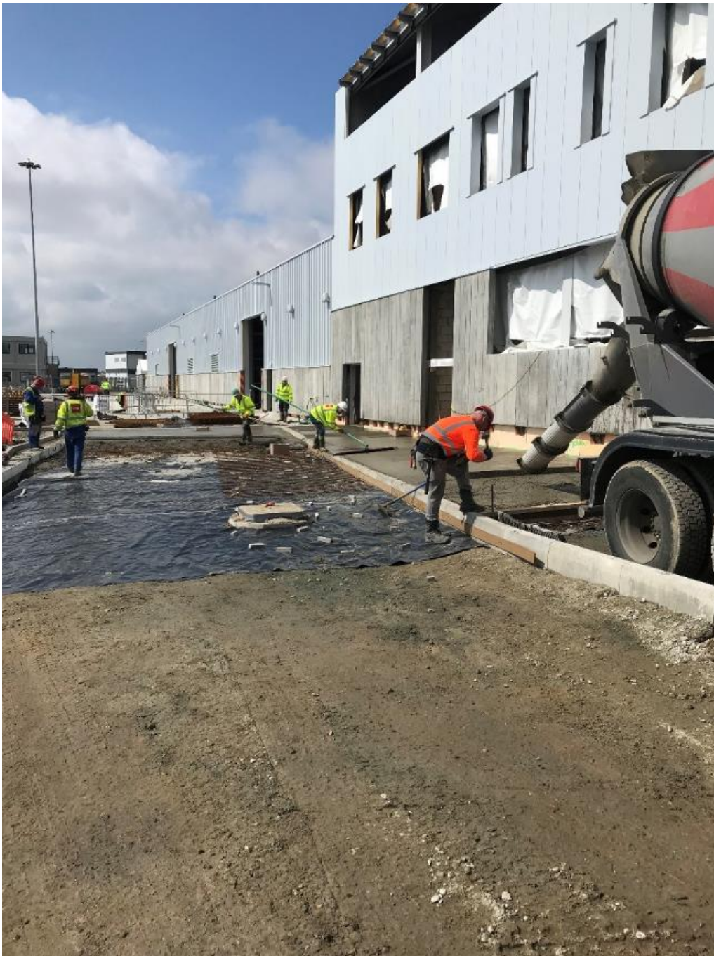
Plate 6.28 Construction of Substation Operational Access Road (example taken from East Anglia ONE substation)
