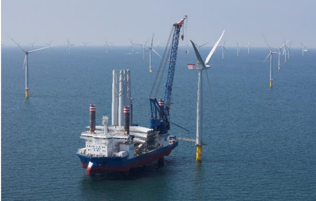
Plate 6.16 Wind Turbine under Construction (photo taken from West of Duddon Sands offshore windfarm)
