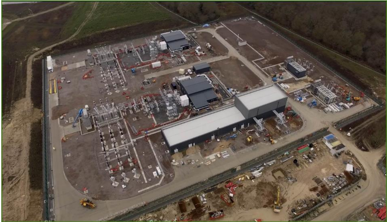
Plate 6.26 Example Layout of the Onshore Substation (example taken from construction of East Anglia ONE substation)
