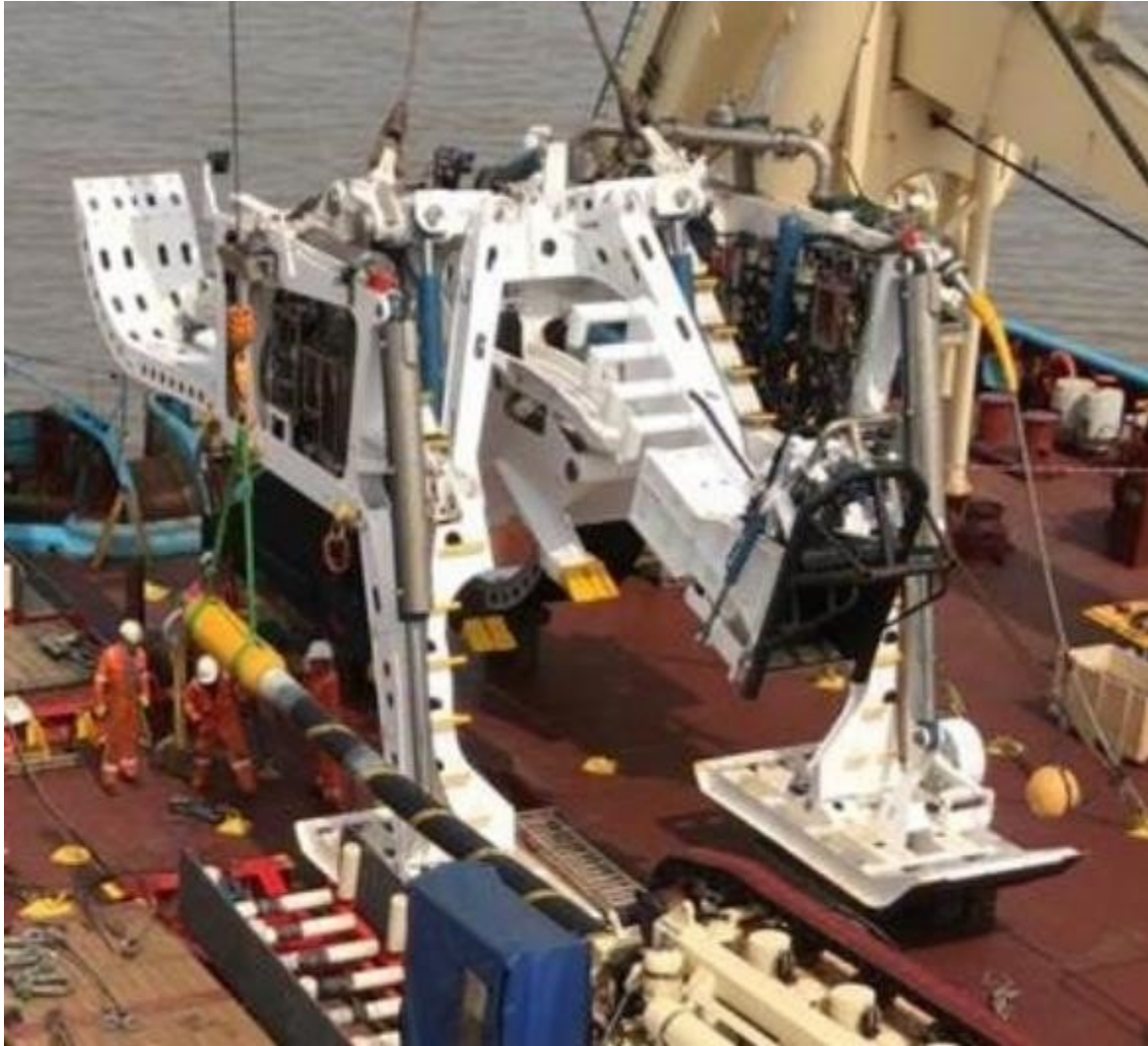
Plate 6.13 Plough which was used to install the offshore export cables at the East Anglia ONE project
