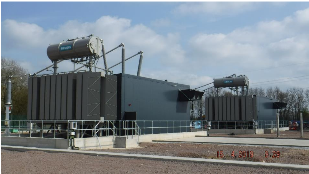
Plate 6.25 Example of Shunt Reactor Building to House Reactive Compensation Equipment (example taken from East Anglia ONE substation)
