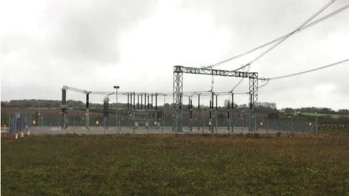
Plate 6.30 Example of Cable Sealing End Compound
